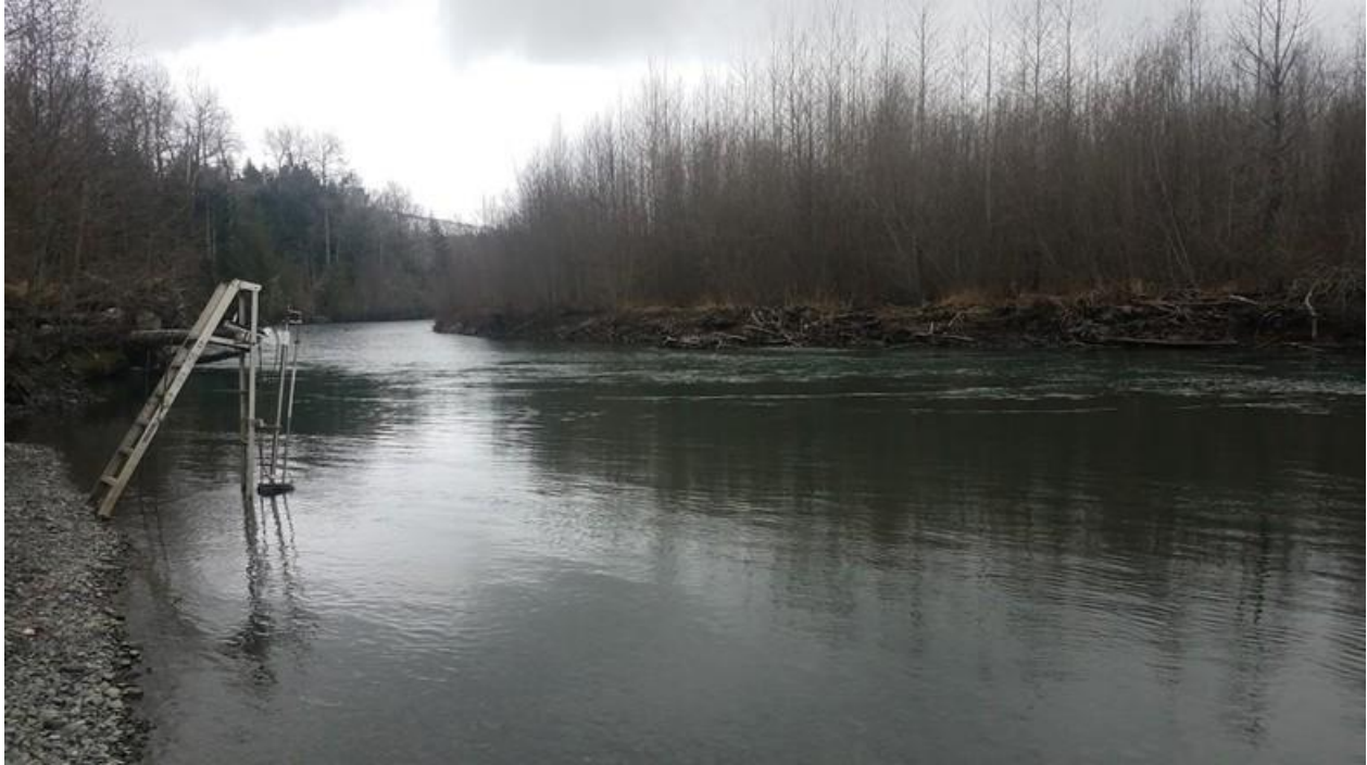
Figure 2. New Old Mainstem SONAR site looking upstream. The SONAR itself is attached to the pole mount which is in turn attached to the ladder. The solar panels and top side box are just out of sight on the logjam in the upper left-hand corner of the picture. The SONAR was operational at this site from June 11 through July 9, 2025.
